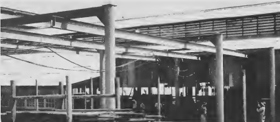
The Pipe Shop (4), formerly (11), is under construction at north side of old shop. The columns and beams shown are a handling structure to move pipe lengths from outside into threading and cutting machines.
